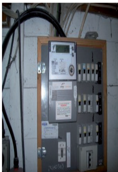
The image above shows a “smart meter” in an industrial building.
